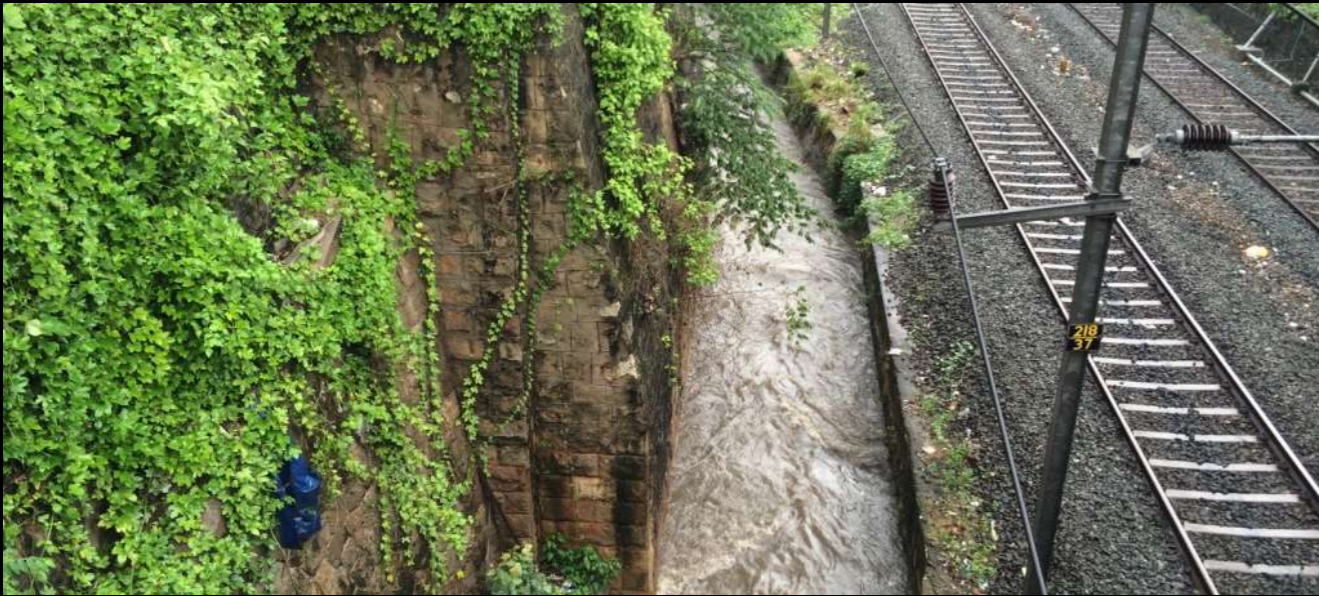
Drains constructed for Overbridge juts into Drains - reduces width
